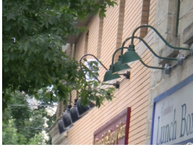
Energy efficient exterior lighting
