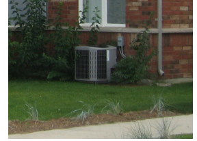
Energy STAR HVAC features
